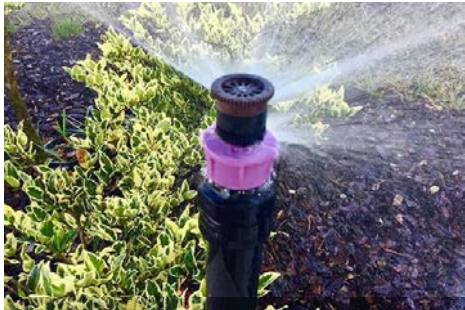
Sprinklers that are purple represent reclaimed water
